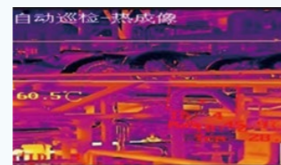
Thermal imaging inspection system
